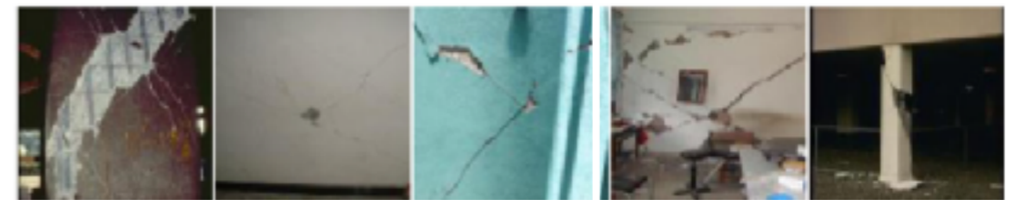
(c) Shear damage
