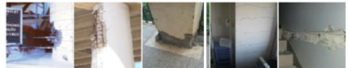
(b) Flexural damage
