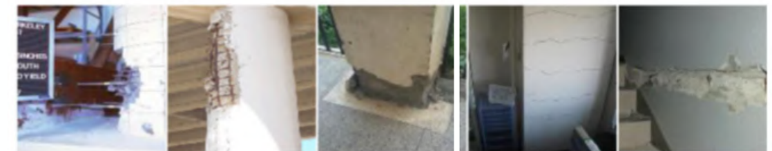
(b) Flexural damage
